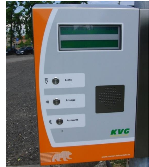
Regio-DFI-Anlage in Seehausen
